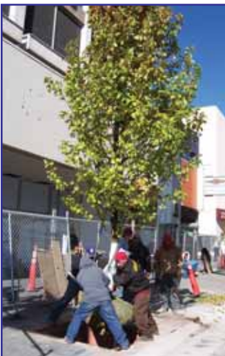
NEMO Nevada supported a project to include four filter boxes in downtown Reno.
