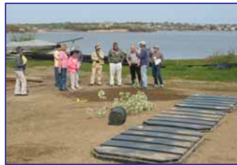
Having knocked over potted trees in their haste to get a first-hand look at newly installed alternative wastewater technologies, NEMOids pay rapt attention to peat filter system operation and maintenance. This demonstration site is located in Charlestown RI.
