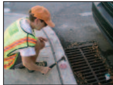
Anne Kitchell, volunteer project coordinator, demonstrates the installation of a storm drain marker in Beaufort, South Carolina. (Photo courtesy of SC NEMO.)
