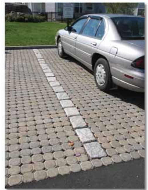
Public access parking stalls at Cornfield Point, Old Saybrook, Connecticut feature alternative pavement that promotes infiltration. Shown here are modular concrete pavers.
